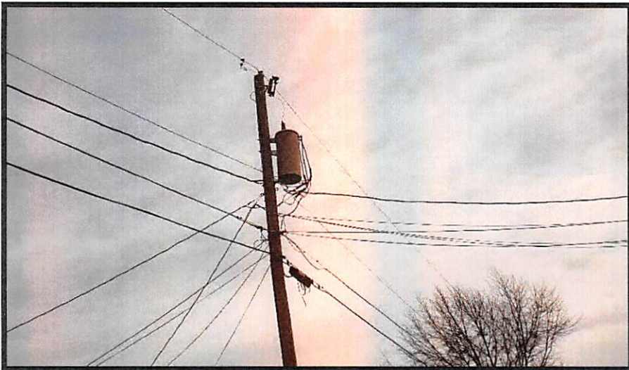
1 of 9 pole-mounted transformers. Owned by Canton public utilities.
